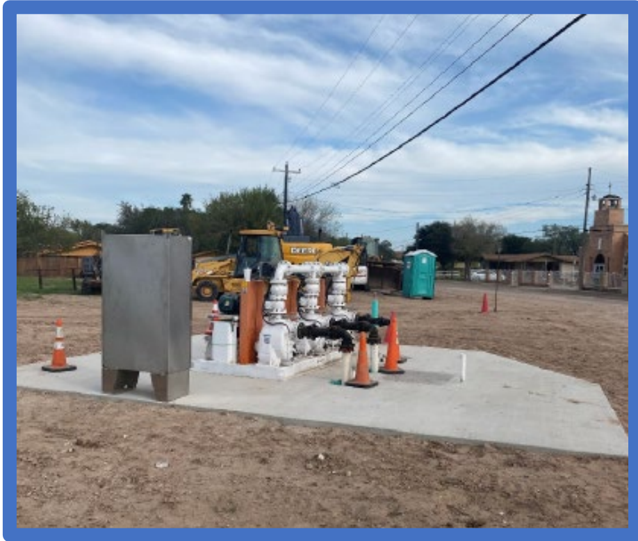
Rio Grande City, Texas installed a new Lift Station with backup pump at their facility, 2019
