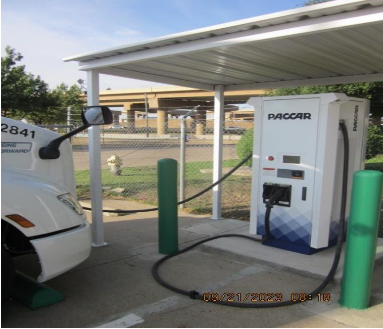
Truck Docked to Charging Unit
