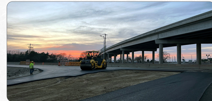
Crews put finishing touches on the initial phase of Loop 9, which opened in late January.
