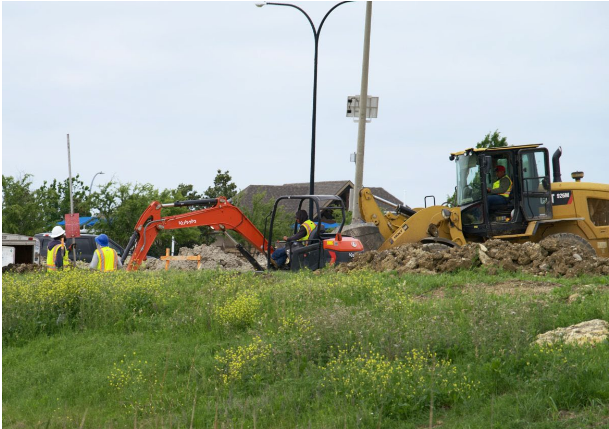
An excavator digs up dirt as workers watch at a building site where new homes are under construction on April 14, 2023, on the corner of Harmon Road and Heritage Trace Parkway in north Fort Worth. (Jacob Sanchez | Fort Worth Report)
