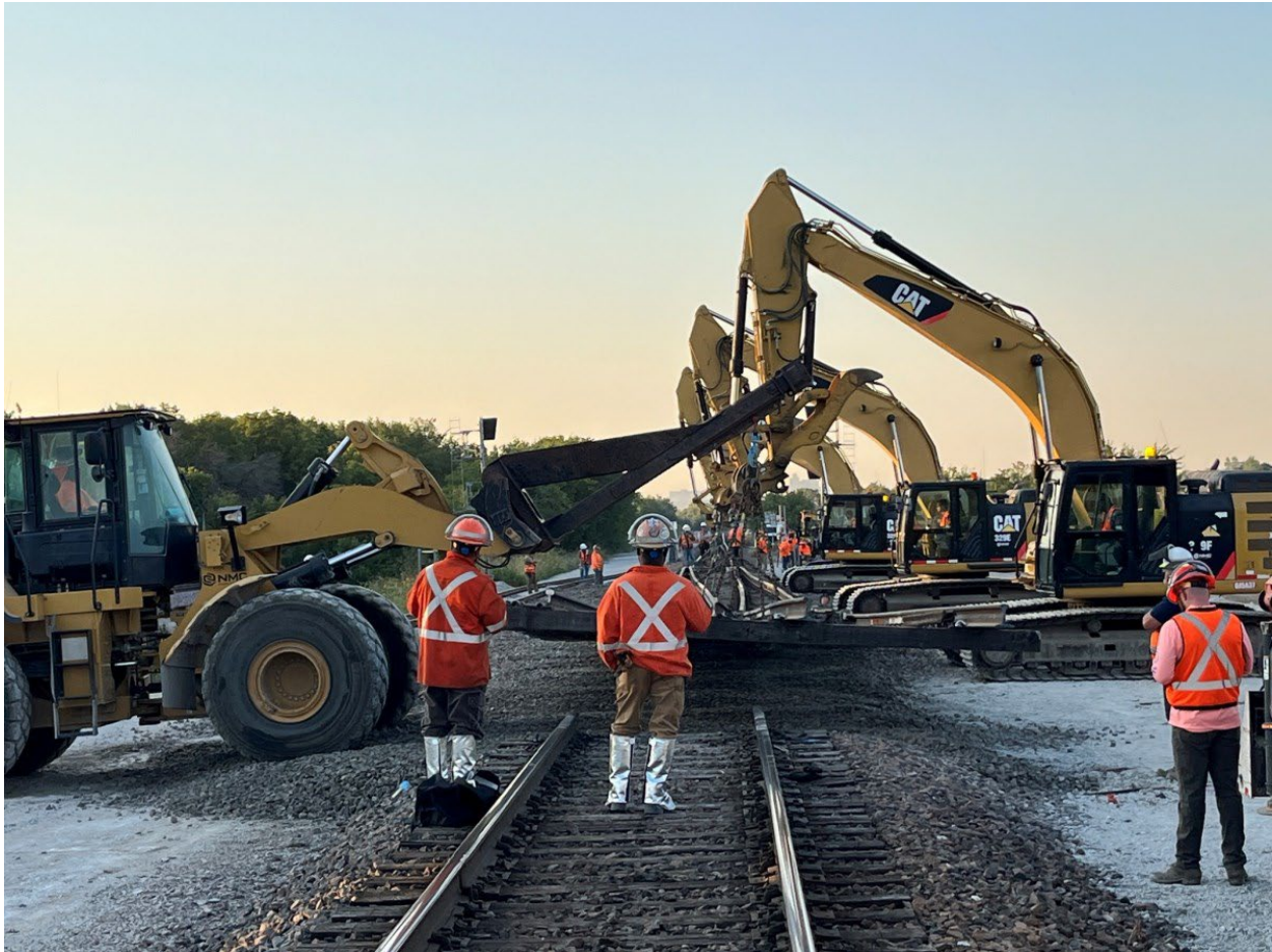
BNSF Railway workers complete a portion of double railroad tracks, a project that will increase capacity in the Alliance area and throughout the state. (Courtesy photo | BNSF Railway)
