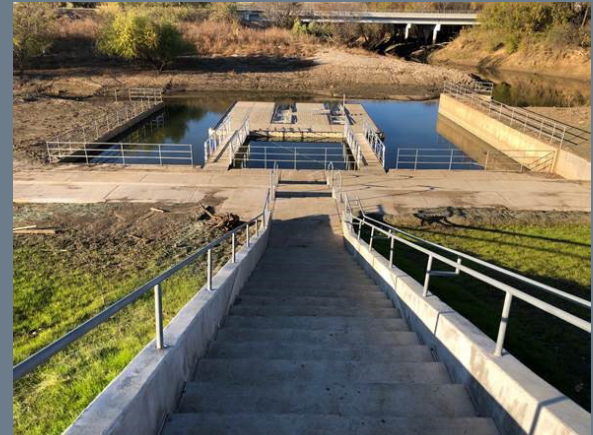
Figure 4.7: The launch site at Lewisville Kayak Launch at Hebron Parkway.
