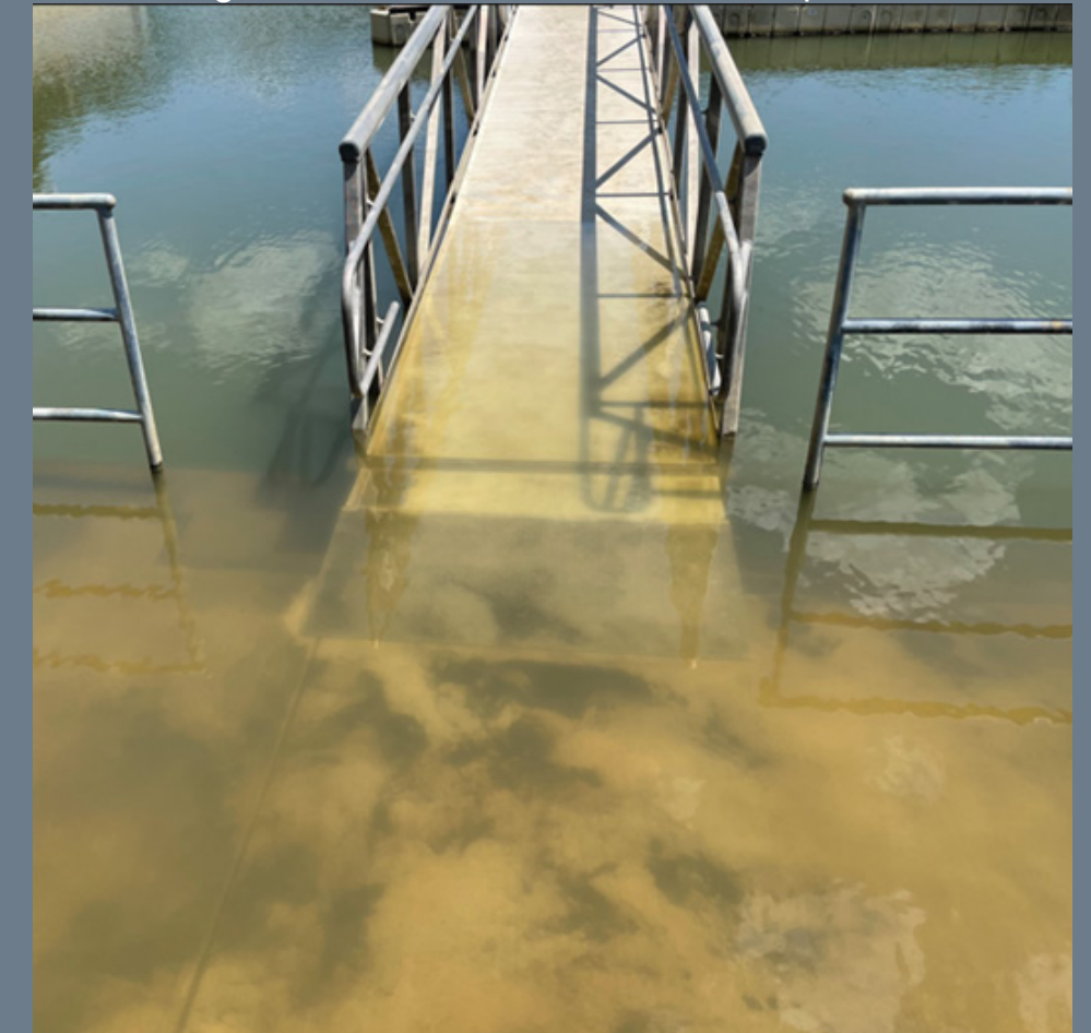
Figure 3.3: Gangway and concrete bulkhead become submerged around 3,000 to 4,000 cubic feet per second.
