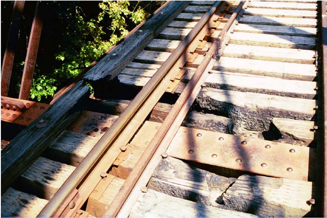
MP 741.1 – Second set of burned ties on Trinity River Bridge
