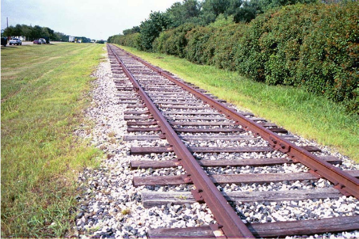
Track out of service just South of Spring Creek Parkway
