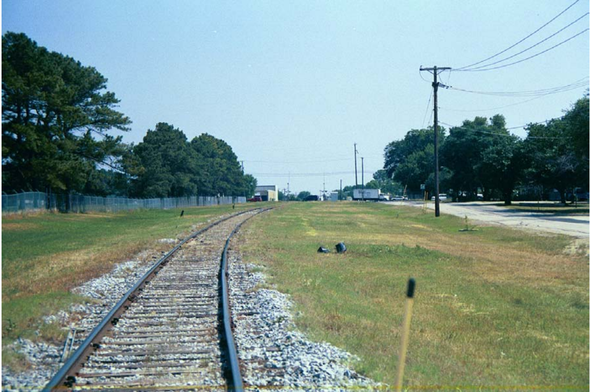
MP 743.5 – Whitlock Lane in distance. Note lack of drainage along track.
