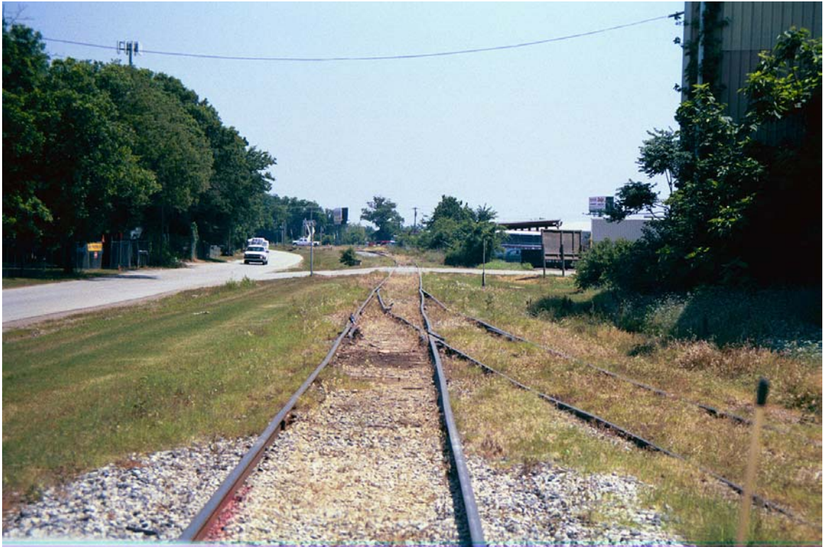
MP 736.9 – South end of siding serving Andes Metal with private road crossing in distance. Note poor track condition.
