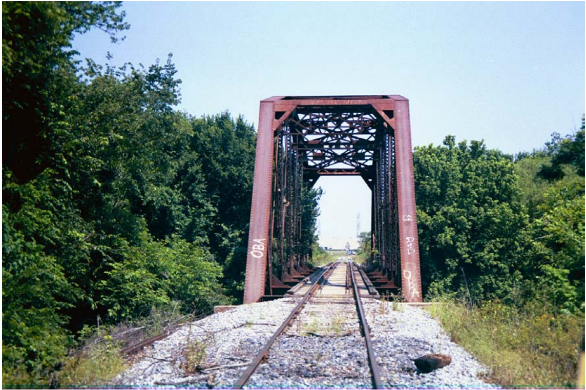
MP 741.1 – Trinity River Bridge consists of 175' long steel truss and 126' long timber pile trestle
