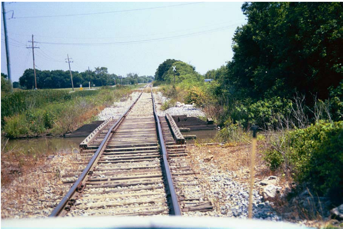
MP 738.3 – Note poor track condition. Bridge is one of four within 0.3-mile and is 39’ in length. Bennett Lane is in distance.
