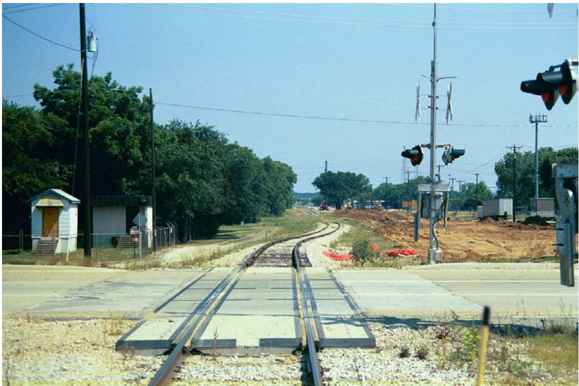
MP 742.4 – Old Trinity Road. Note curves in track resulting from new bridge alignment.
