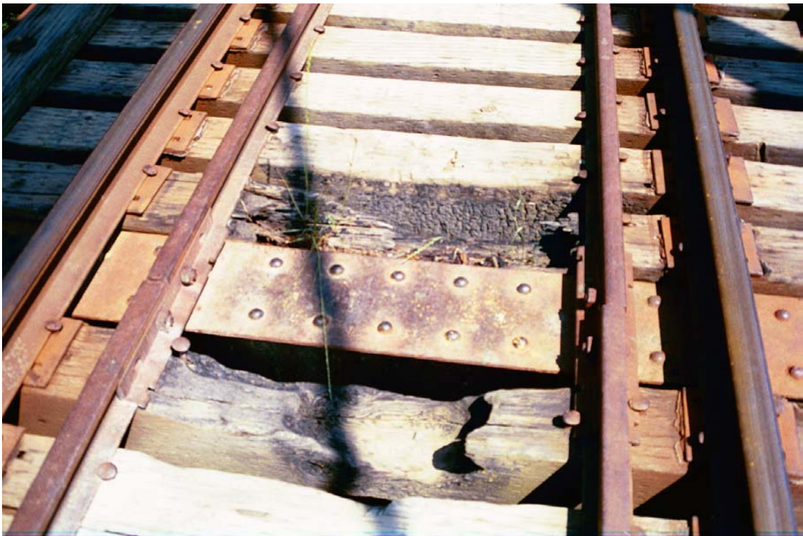
MP 741.1 First set of burned ties on Trinity River Bridge
