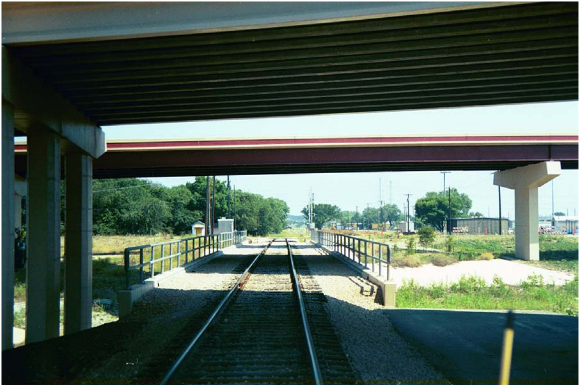
MP 742.4 – Bridge under SH-190 overpass is 112 feet in length. Old Trinity Road is in distance.
