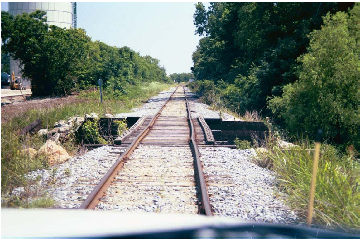
MP 736.3 – Bridge is 42' in length. Note very poor track conditions
