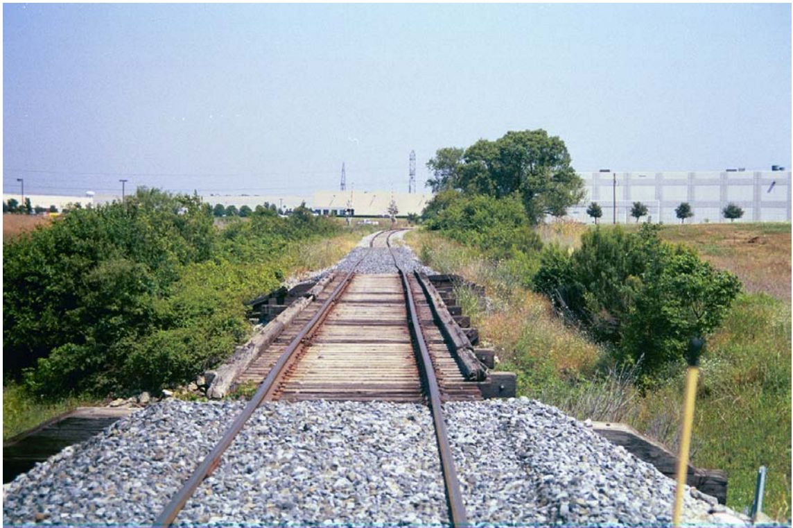
MP 741.2 – Bridge over Elm Creek is 104' in length and is just south of the Trinity River Bridge.
