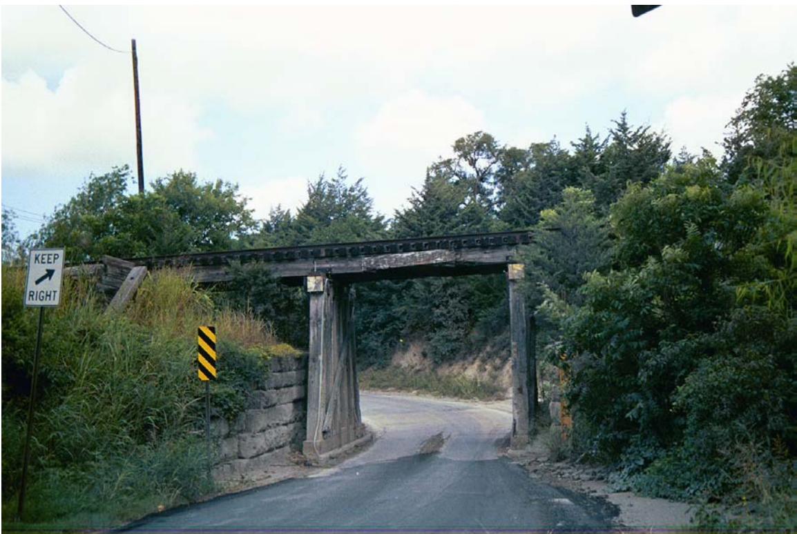
Old Mills Rd Historic Overpass (leads to land fill site) Looking West
