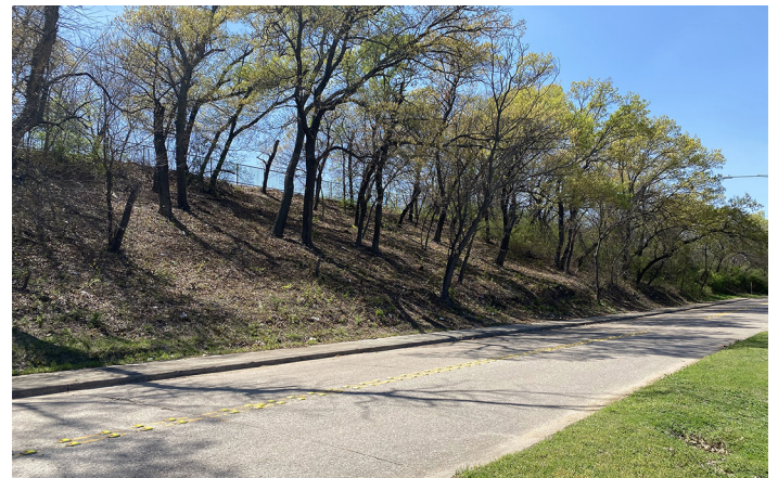
Existing erosion on slope
