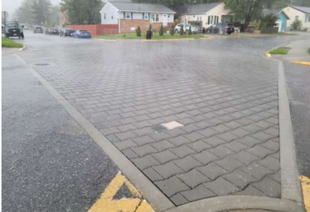
Installation of permeable pavers in traffic intersection in Maryland. The pavers pictured above are capable of supporting AASHTO HS-25 truck loading .
