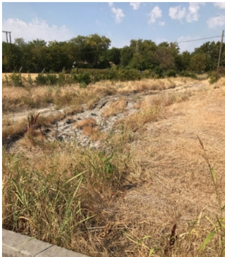
Photo: Silt deposits filling drainage ditch
