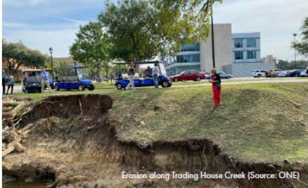
Erosion along Trading House Creek (Source: ONE)
