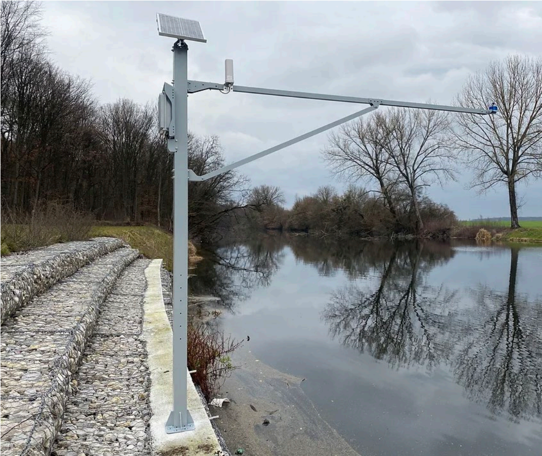
Side of River Installation
