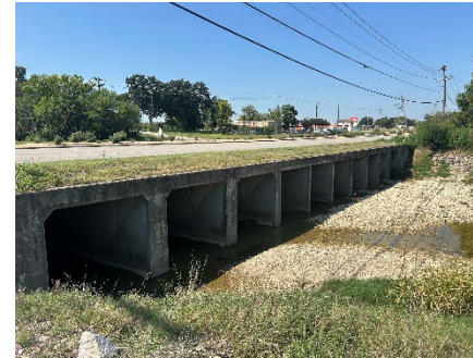
Limited undercrossing clearance at Hurst Boulevard and Calloway Branch Creek.
