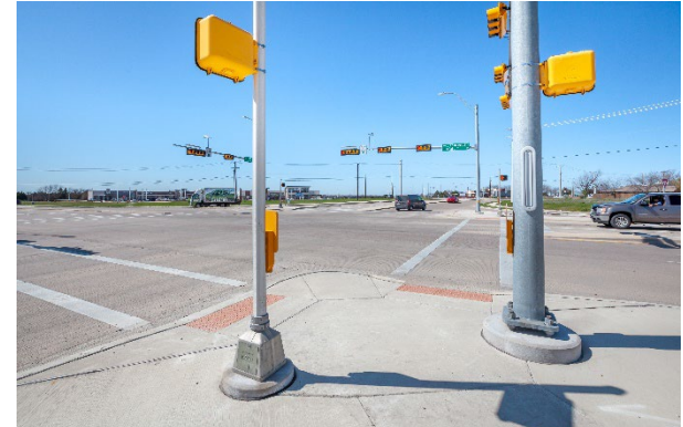
Example of an intersection with aligned curb ramps and pedestrian signals in close proximity for ADA accessibility.
