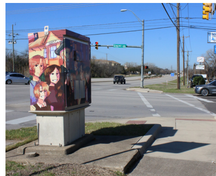
Traffic signal control box with public art at the intersection with Precinct Line Road.
