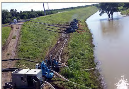
TxDOT crews pumping tens of millions of gallons of water back inside the levees of the Trinity River and off of State Loop 12.
