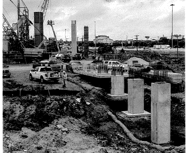
Bridge column construction on the I-30/SH 360 Interchange Project in Arlington. The $233 million project will increase safety, connectivity and mobility for motorists.
