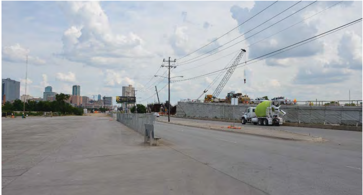
Figure 12. Typical Industrial Frontage Near SH 199 and West Fork of the Trinity River Bridge
