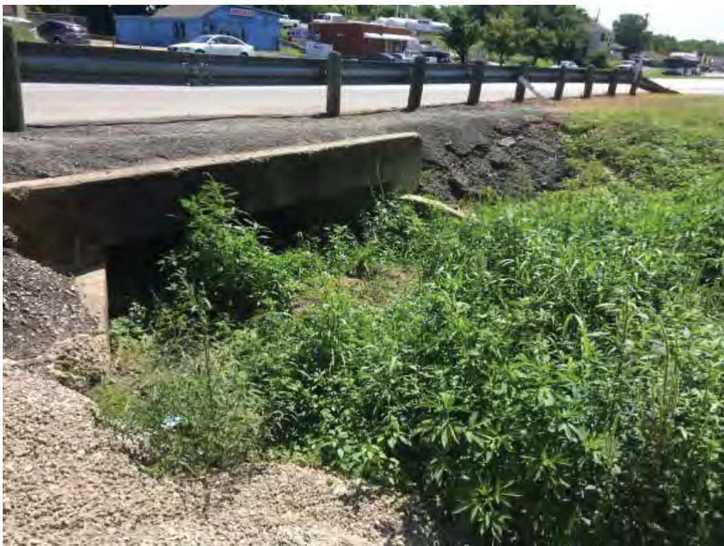
Figure 2. Silted Culvert (SH 199, Sansom Park) Source: Freese and Nichols, Inc., 2016
