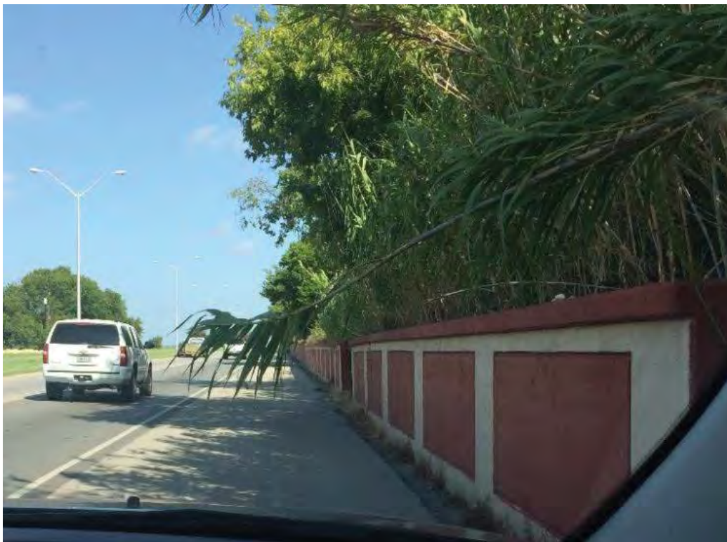
Wall Blocking Drainage at Jacksboro Highway; No Curb and Gutter
