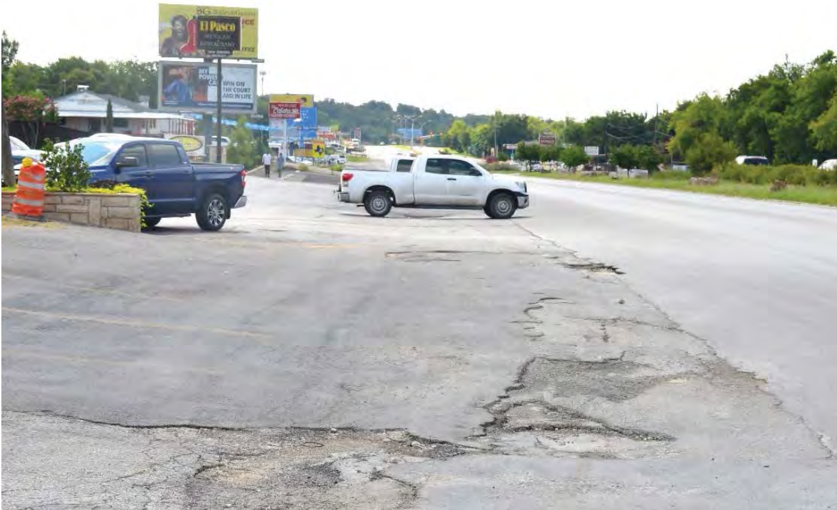
Figure 9. Private Development Obstructing Intersection Sight Distance Within TxDOT ROW East of SH 199 and Trails End Street Intersection
