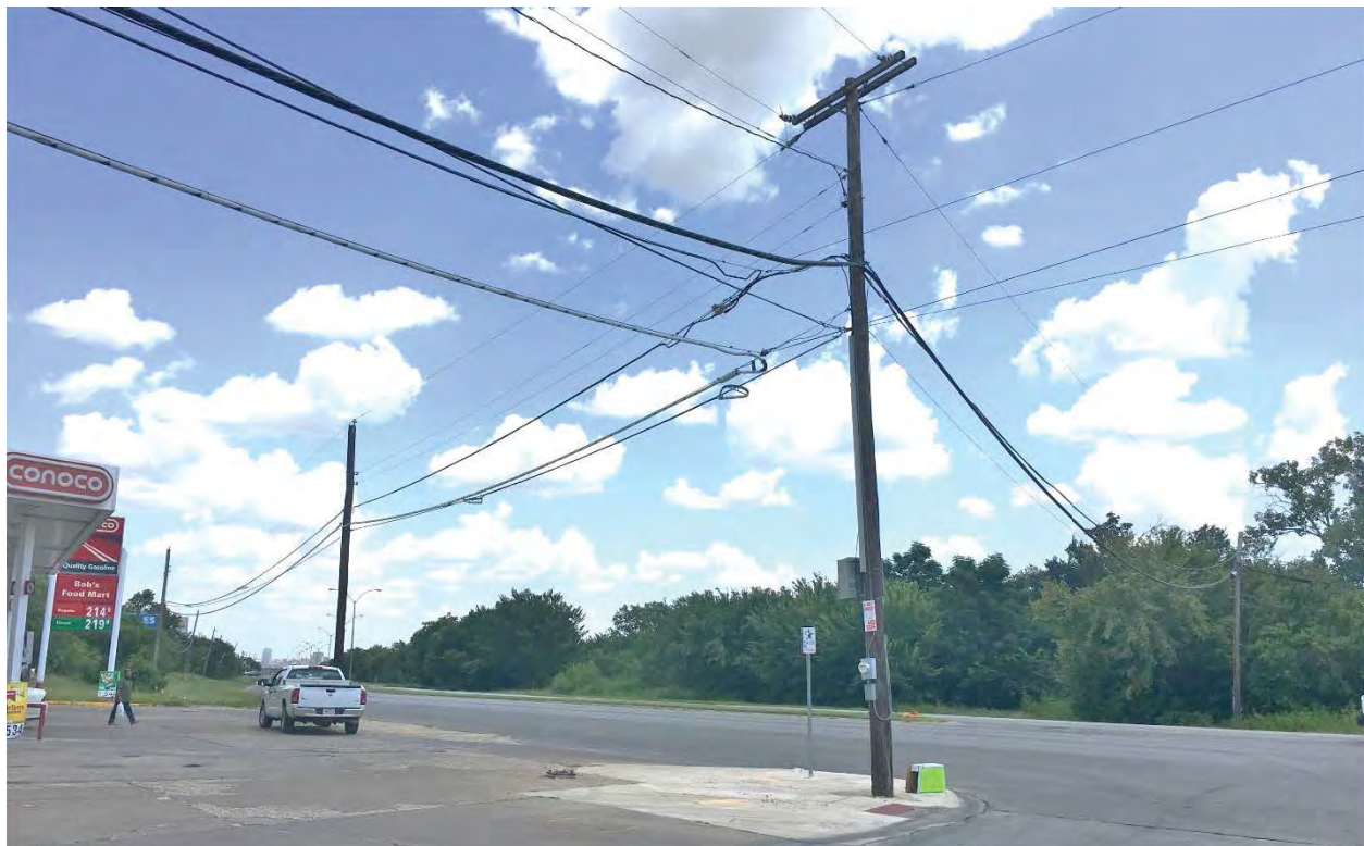
Figure 2. East Perspective of Overhead Utilities East of Skyline Drive Source: Freese and Nichols, 2017
