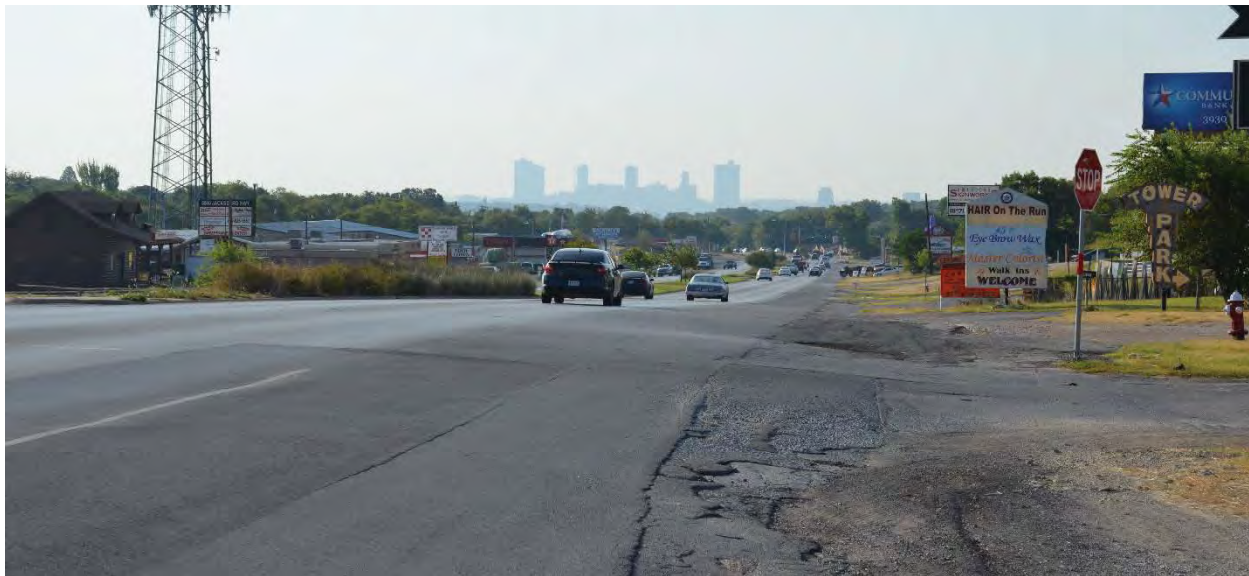
Figure 11. Existing Pavement Conditions Along SH 199
