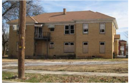
Dilapidated Multifamily Housing
