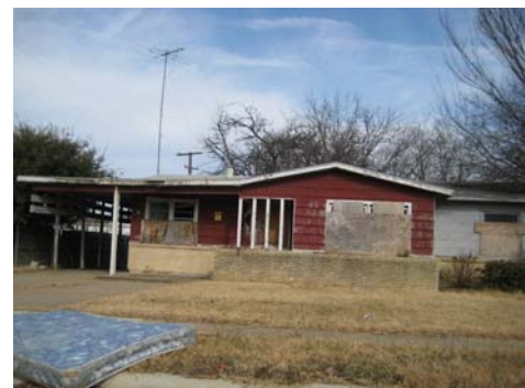
Dilapidated Single-Family Housing
