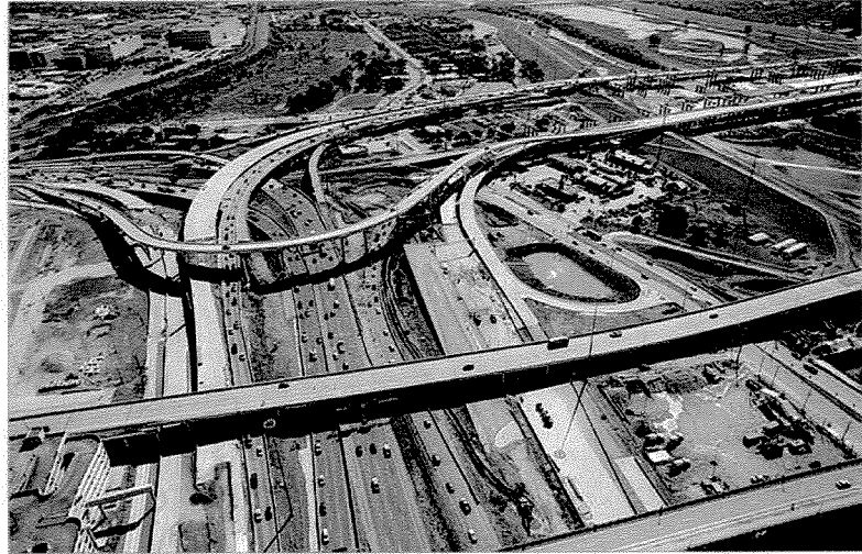
Pictured above is an aerial view looking east toward the new bridge carrying westbound I-30 traffic to southbound I-35E. This traffic switch occurred on October 26, 2015.
