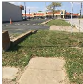
Sidewalk Gaps on Floyd
