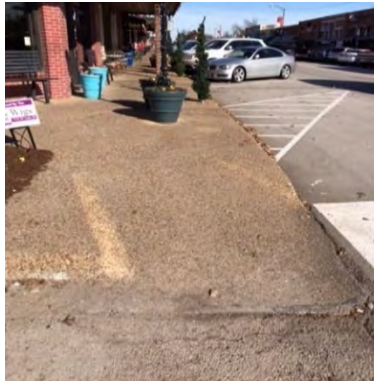
Curb ramp on Ballard Avenue not meeting best practice standards
