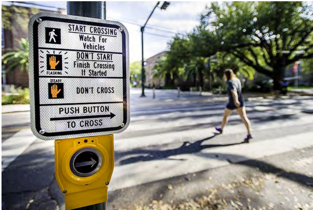
Figure 11. Accessible Pedestrian Signal Pushbutton Assembly
