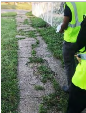
Heavily cracked sidewalk on Bentley Ave. in front of Cowart Elementary.
