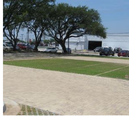
Figure 19. A parking lot installation of permeable pavers in Carrollton, Texas. Source: City of Carrollton.
