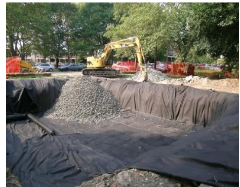
Figure 69. A subsurface infiltration bed under construction at Clark Park, Philadelphia, Pa. Source: Philadelphia Water Department.
