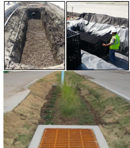
Figure 32. The construction of bioswales in the median on Merritt Road, Rowlett, Texas.
