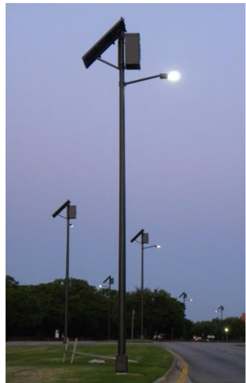
Figure 4. The City of Irving's solar streetlight.
