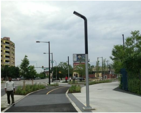
Figure 5. Solar lighting installation on Penn Street Trail, Philadelphia, Pa. Source: Delaware River Waterfront Corporation.
