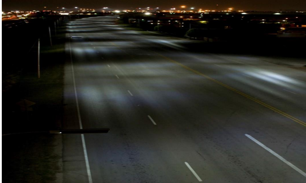
Figure 1. Main Street, Grand Prairie, after LED installation. Source: Oncor, 2012.
