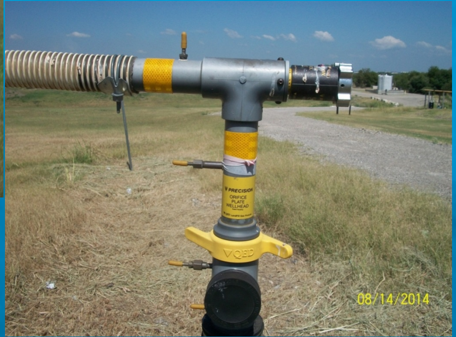
Landfill gas wellhead
