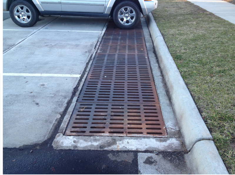
Sand Filter Drain in Raleigh, NC. Source: Tetra Tech
