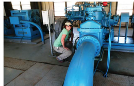
Sampling at Moss Creek Lake Pump Station
