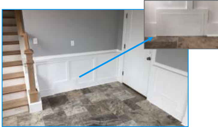
Pictured: Foyer application meets 2018 Energy Codes
