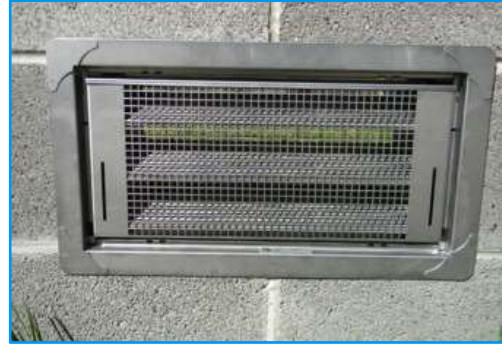
Flood door closed, obstructing the opening.
