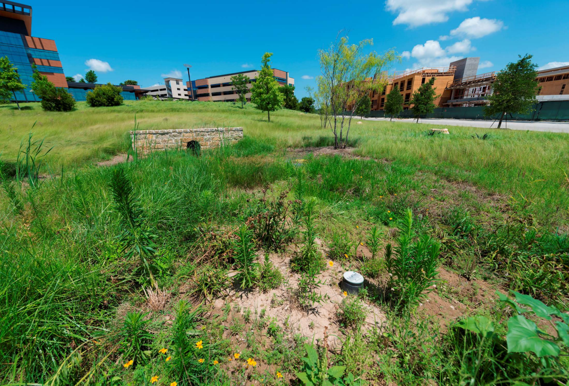
Maintenance Issues: Plants & Mulch
